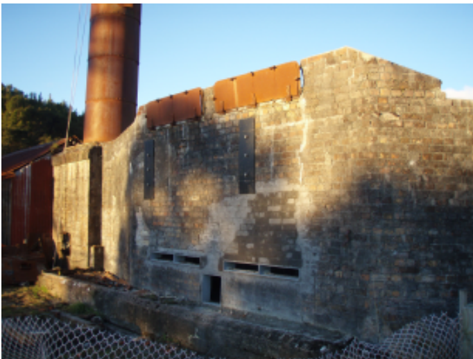
Below: Restored brickwork and steelwork on the South Shaft flue where there'd been a large gap for more than half a century.
