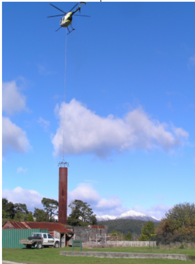
Placing a steel mesh on the South Shaft chimney before renovation work. A safety barrier suspended from the mesh was to prevent anyone working down in the flue from getting crowned if any of the brick lining in the chimney came loose. Nothing did.
