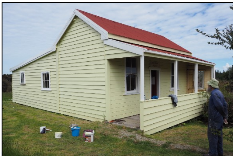
A satisfied Paul surveying the finished side of Gills Cottage. This involved weatherboard replacement and painting. There are two sides to go.
