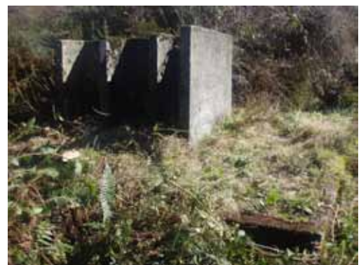
The toilet block near the Rec, with the concrete floor in the foreground and the cubicles silhouetted in the bright Waiuta sunshine.
