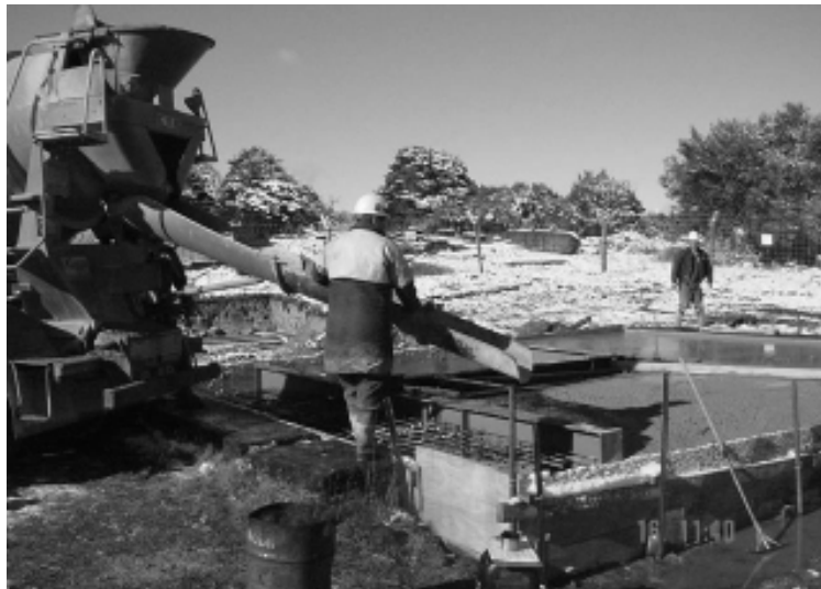
Pouring concrete for the new headframe foundations at the Prohibition shaft. The white stuff in the background isn't concrete, but snow. (Photo courtesy OGL.)
